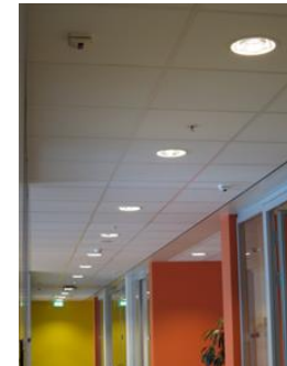
Philipps Lighting Test Bed in Eindhoven
